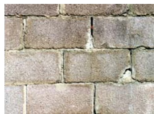
Mortar Joint Deterioration
