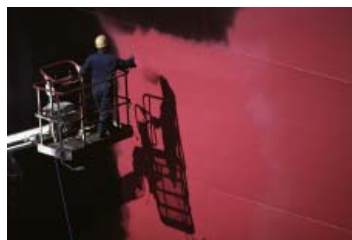
Outdoor metal tanks
