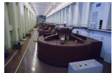
Mechanical equipment rooms
